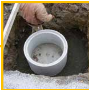
Customer-side concrete ring
