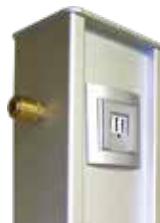
Compressed air and data socket
