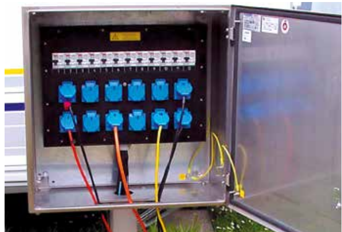
Wall mounted distributor
