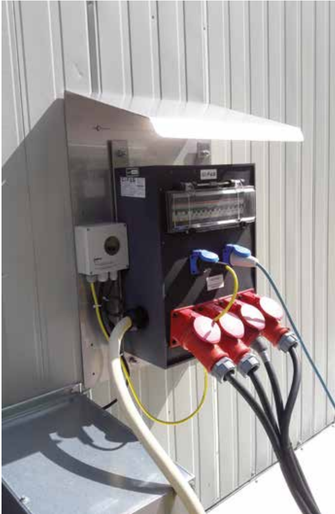
Wall mounted distributor
