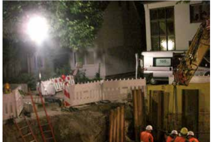
Construction site lighting
