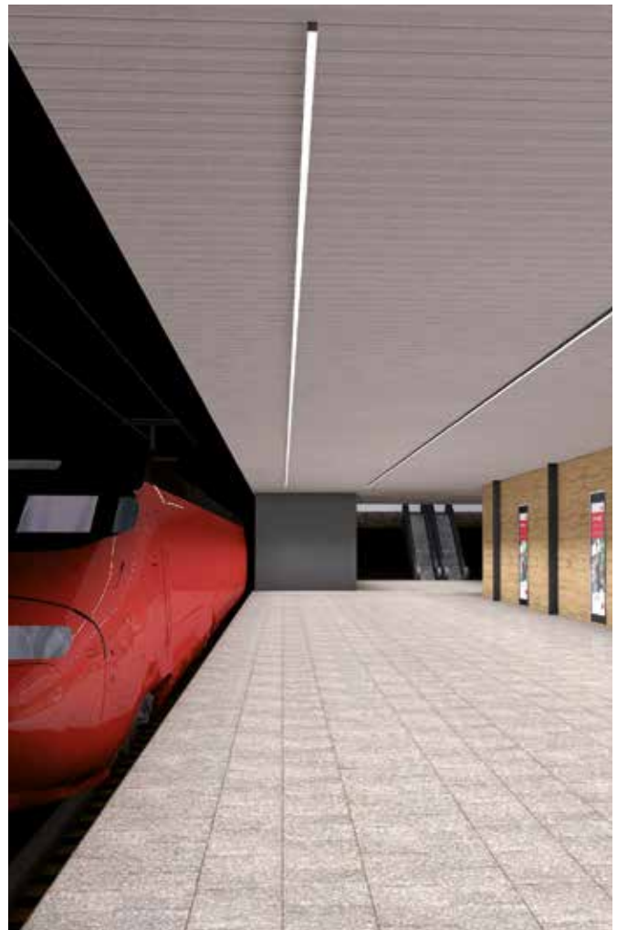
Ceiling lighting for railway station
