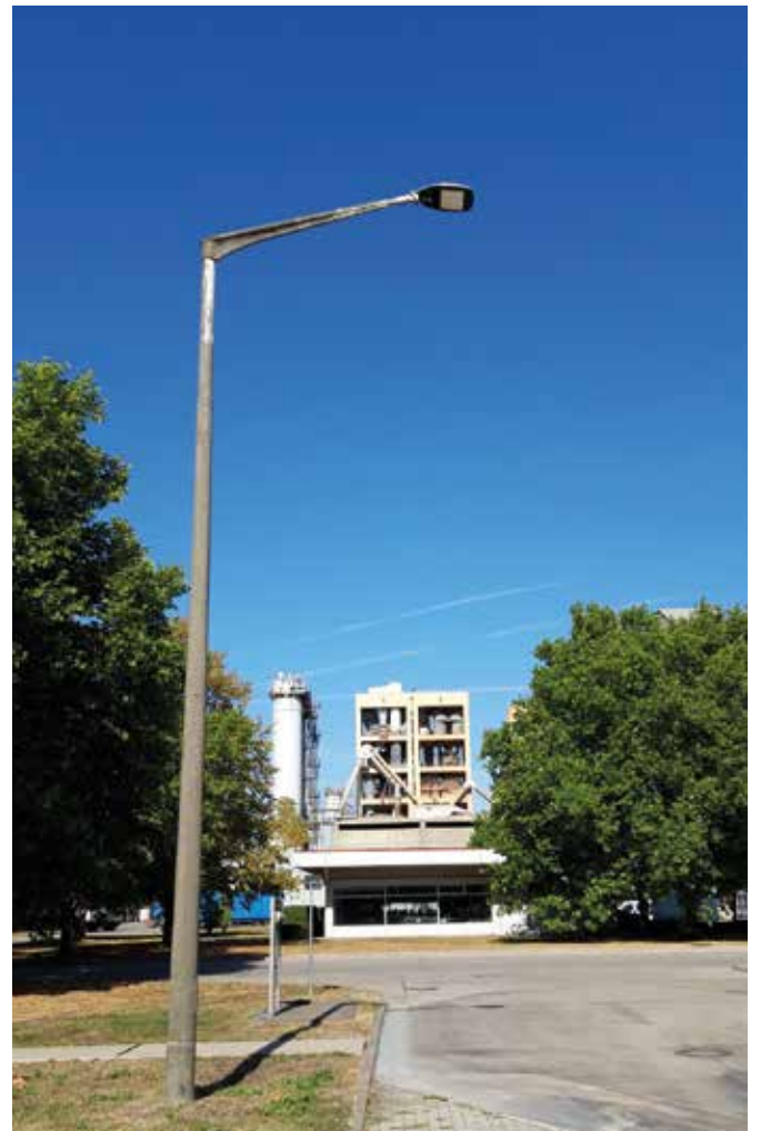
Parking lot lighting, Göllheim
