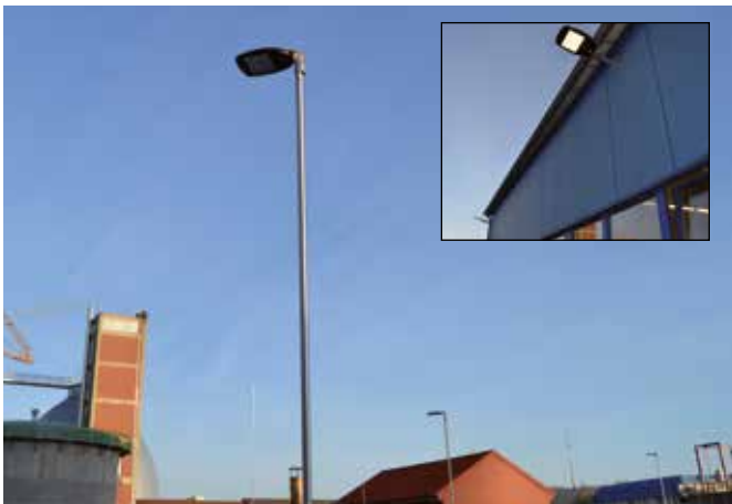
Sewage treatment plant, Osnabrück
